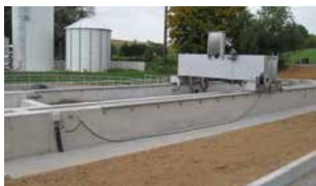
▪ HIK Sandfangräumer / HIK sand trap scraper
